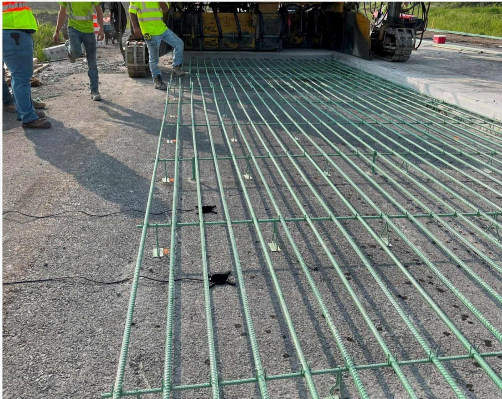
Drop on Roadbed
